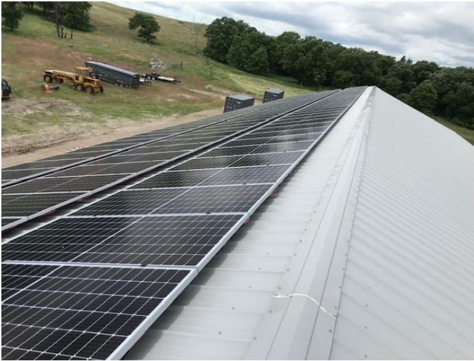
The solar array at the Niobrara Valley Preserve. Photo © Randy Schantell/SWT Energy
