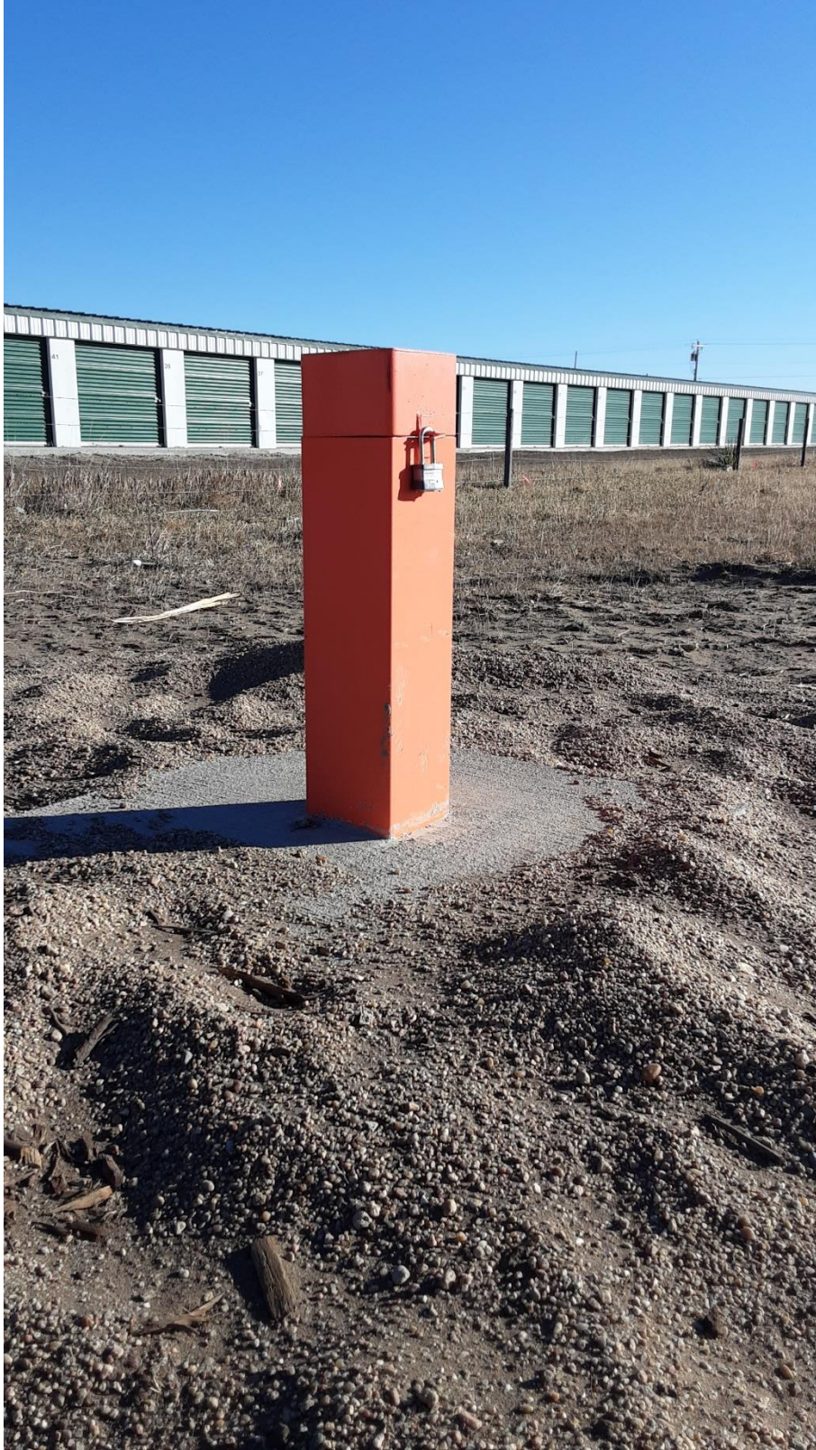
One of Three dedicated observations wells. All wells have different casing, protective covers, measuring equipment, and technology seen across the state.
