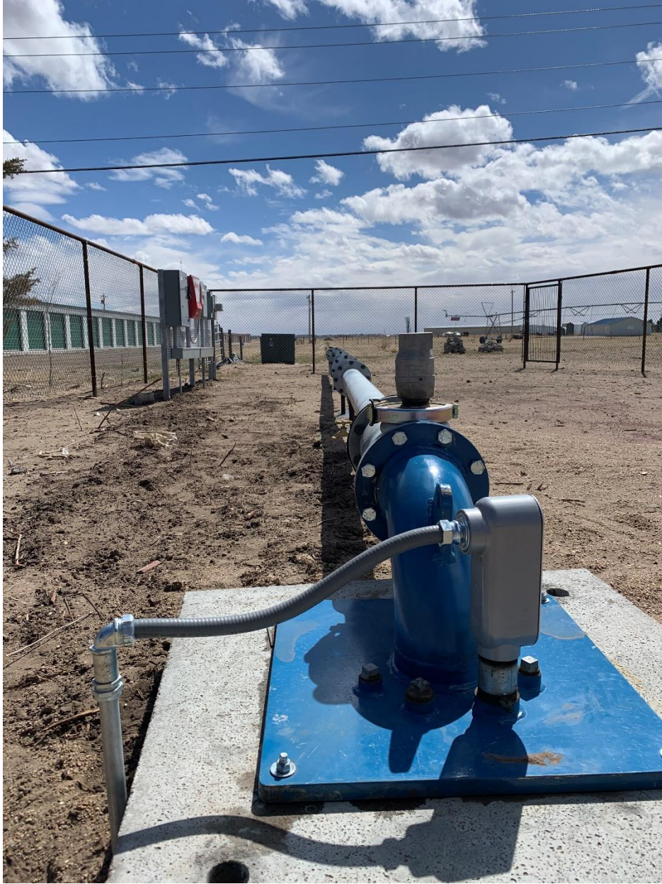
Fully functional irrigation well, multiple spots for flow meters, the newest technology at the panel, and ready for chemigation setups.
